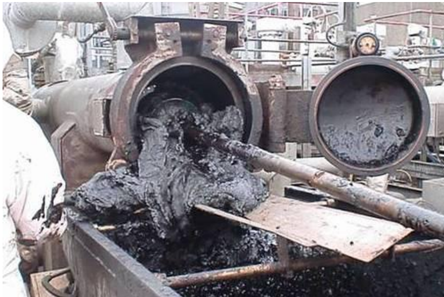
Figure 5: Debris build up within trap after cleaning.
