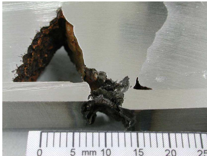
Figure 4. – Corrosion of clad pipeline due to incorrect material used for weld root
