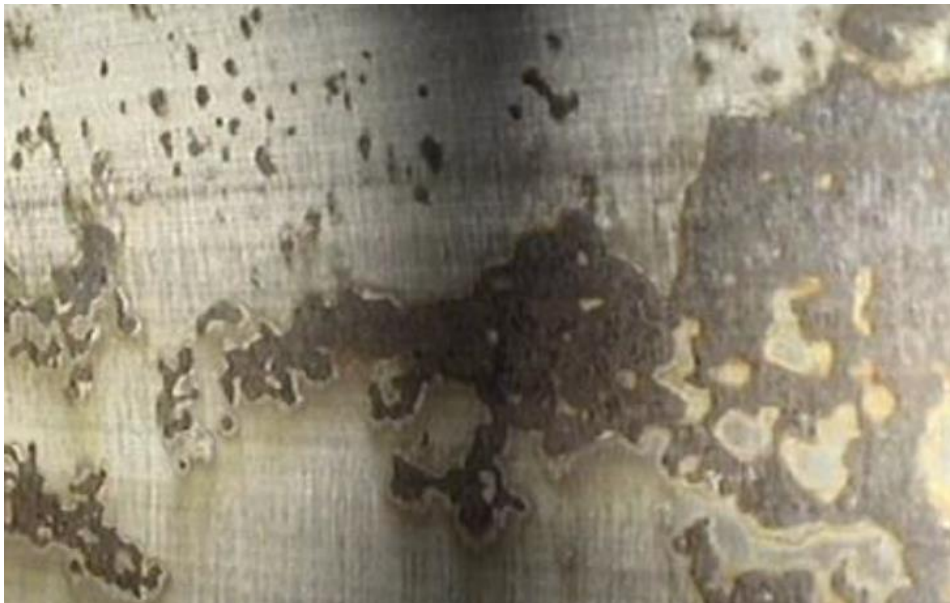
Figure 2. – Example of contamination of CRA surface of lined pipe section
